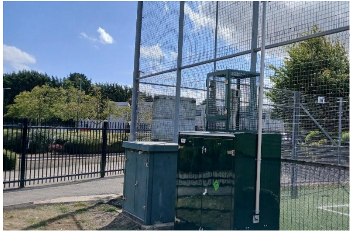
View of AQMS and Inlet Manifold Cage
