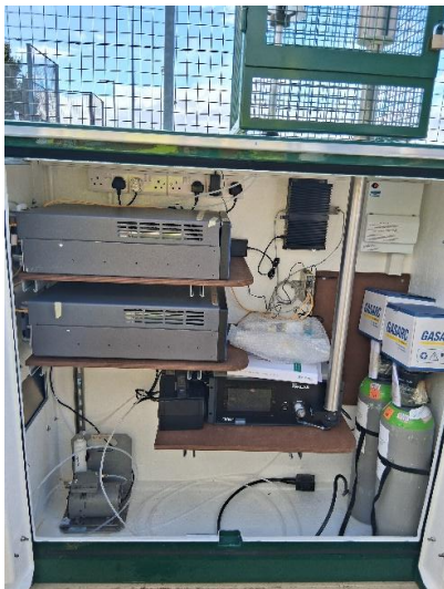
Internal View of AQMS
