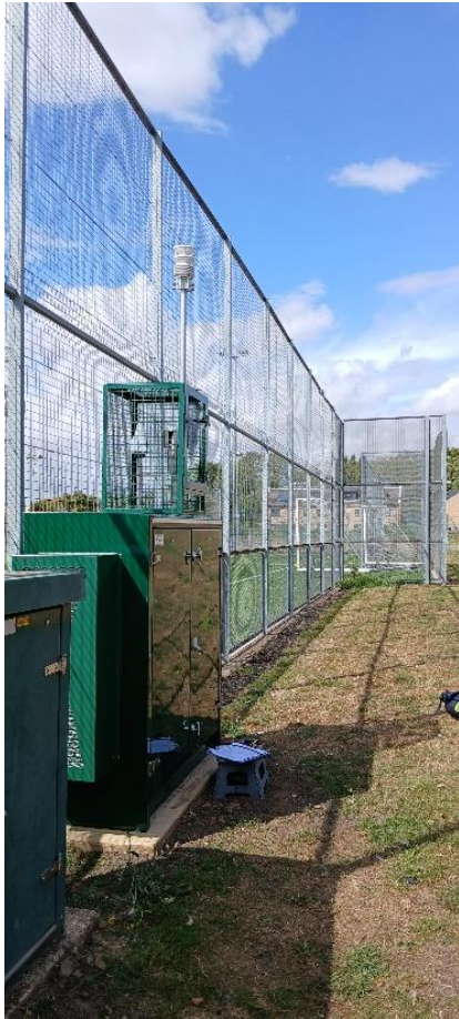
View of AQMS and Meteorological Sensor
