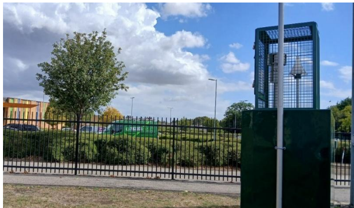
Manifold Aspect of AQMS Inlet Manifold Cage
