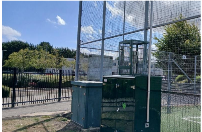
View of AQMS and Inlet Manifold Cage
