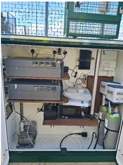
Internal View of AQMS
