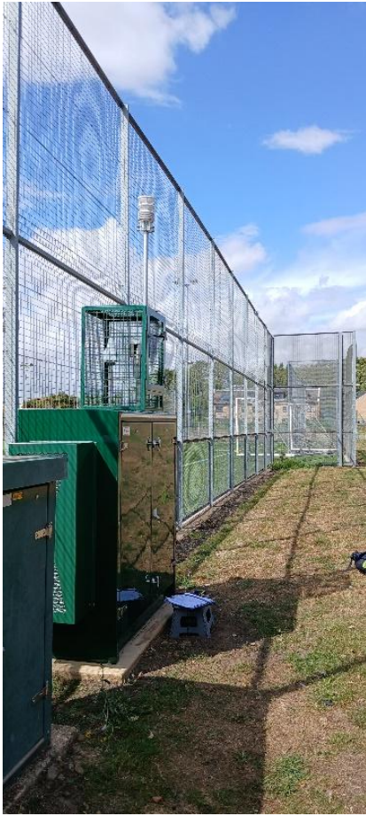
View of AQMS and Meteorological Sensor
