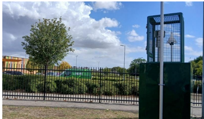
Manifold Aspect of AQMS Inlet Manifold Cage
